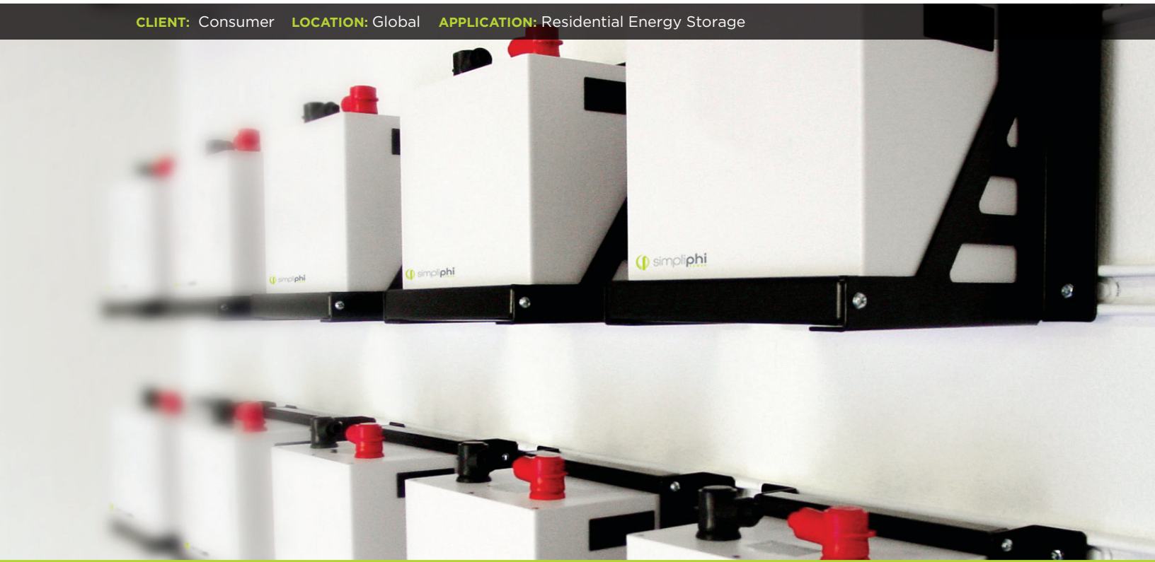
Above: 20 OES2 Smart-Tech Energy Storage Batteries provide 52kWh of power
