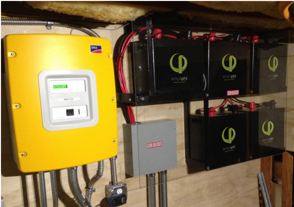
Figure 2.0 - PHI 3.4™ 48 Volt, 60 Amp, Batteries: 17kWh Residential Installation
